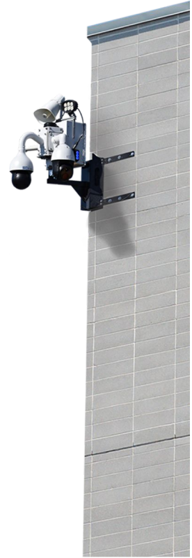
BUILDING AND POLE MOUNT
